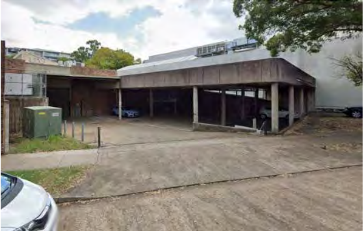
Photo 5: Undercroft area existing on the site that would be subject to inundation in flood events. Source: Google Street View, dated March 2021.
